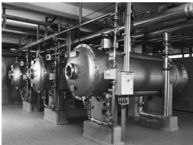
Fig. 4 Ozone generators for water treatment (by courtesy of Ozonia Ltd).
